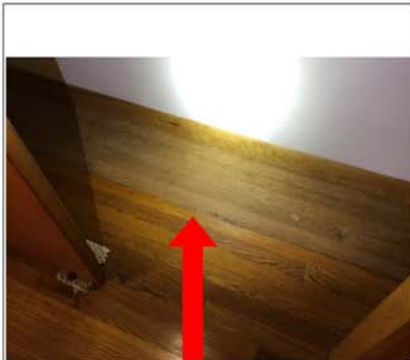
Closet floor some not stained
