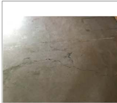
Floor typical cracks
