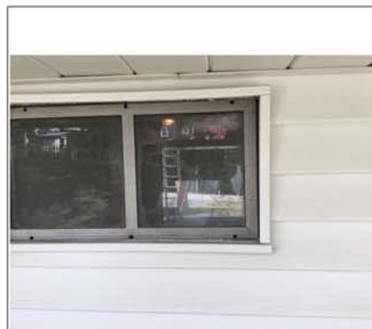
SHED WINDOW CRACKED
