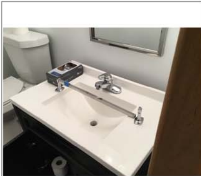
Sink not mounted-hooked up No outlet
