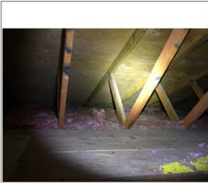
NO BAFFLES AT EAVE VENTS IN GARAGE No baffles in house
