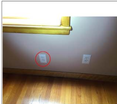
All outlets open/ground except 1 west circled
