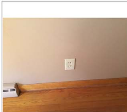
All outlets open/ground
