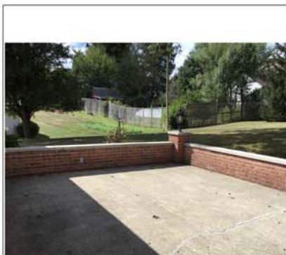
PATIO LIGHTS & 1 OUTLET TRIPS BREAKER
