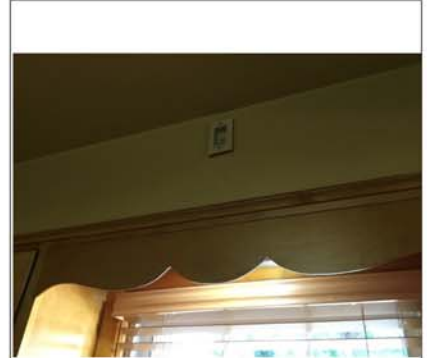
Outlet above sink loose in wall Light cover missing above sink
