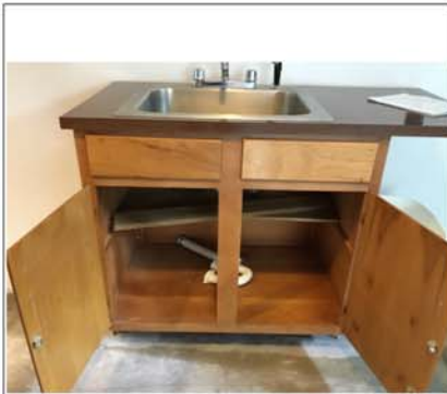
Sink not mounted-hooked up
