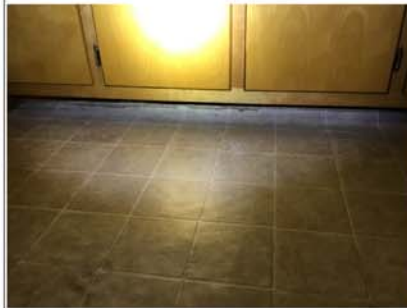
Flooring rolled up under sink cabinet Floor transition strip at door missing
