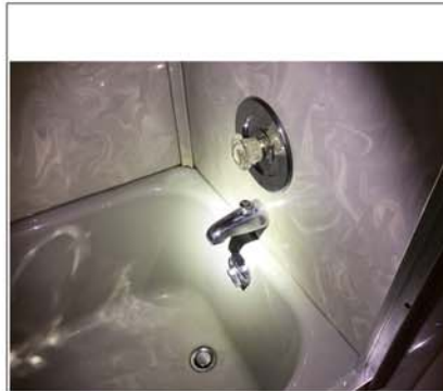
Tub diverter needs adjusted. Water comes out spot-shower at same time
