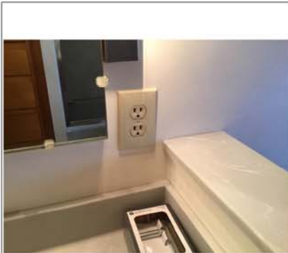
Outlets at sink not GFCI
