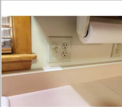
Outlets at sink not GFCI. 1 outlet east wall dining room-south between closet doors-hallway are open/ground.
